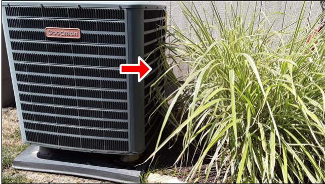
3.0 Item 1(Picture) - Vegetation against A/C condenser
