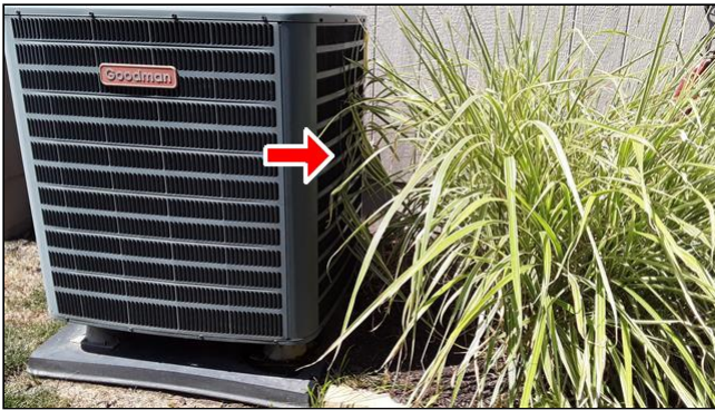
3.0 Item 1(Picture) - Vegetation against A/C condenser
