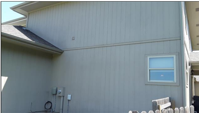
2.1 Item 1(Picture) - Open gaps and exposed nails on North side of home
