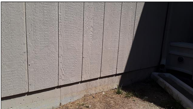
2.1 Item 3(Picture) - Exposed nails at NW corner of home
