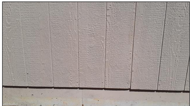
2.1 Item 4(Picture) - Close-up of exposed nails at SW corner of home
