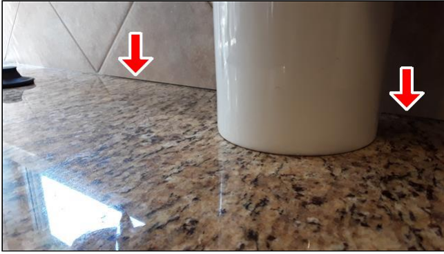
9.8 Item 1(Picture) - Deteriorated grout at kitchen countertop
