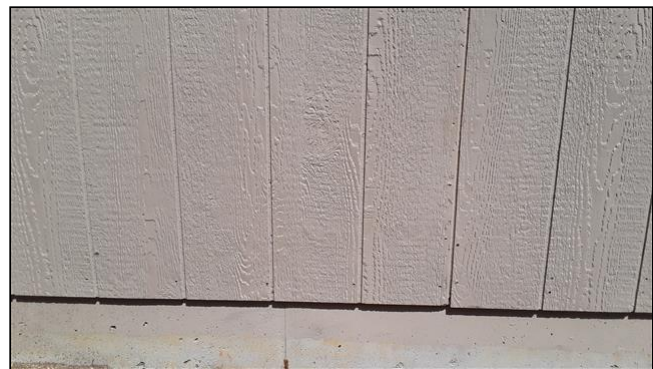
2.1 Item 4(Picture) - Close-up of exposed nails at SW corner of home
