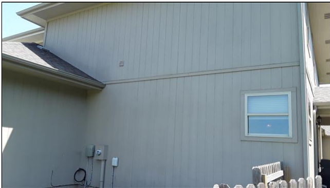
2.1 Item 1(Picture) - Open gaps and exposed nails on North side of home
