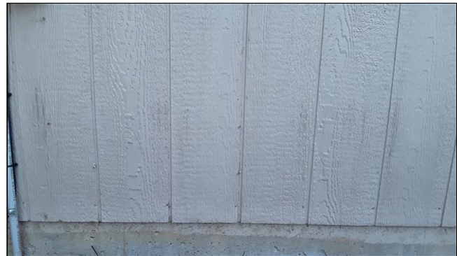
2.1 Item 2(Picture) - Close-up of exposed nails and open gaps on North side of home
