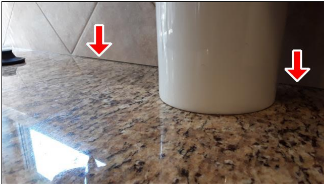
9.8 Item 1(Picture) - Deteriorated grout at kitchen countertop
